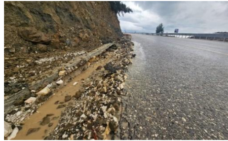
Photo 1. The collapse of surface water channels.
