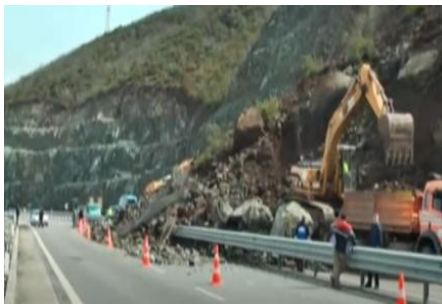
Photo. 1: The landslide of March 24, 2018.
