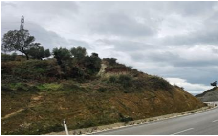
Photo 2. Blockage of the channel leading to water overflow onto the road
