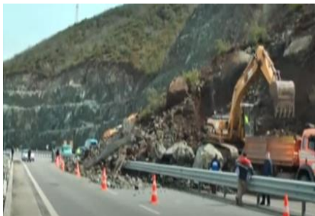
Photo. 1: The landslide of March 24, 2018.
