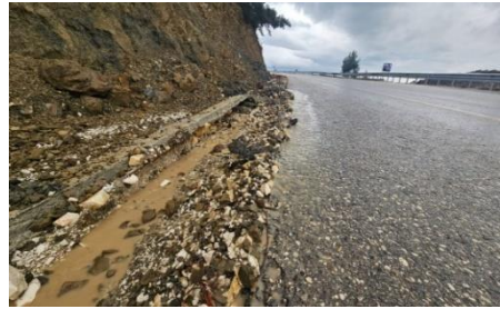
Photo 1. The collapse of surface water channels.
