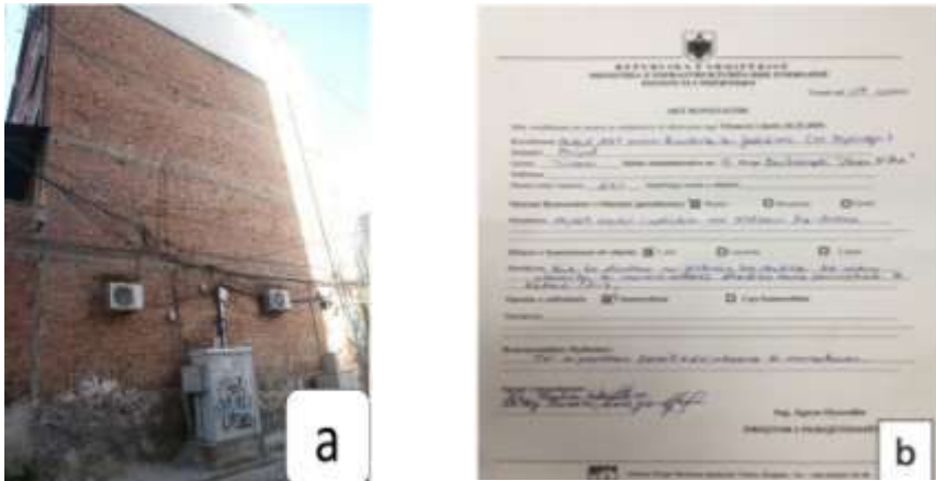
Fig.1: a) Post-earthquake damage assessment, Durres, 2019. Four-storey masonry building in Tirana (common structural system for the city) and, b) General view of a completed form after a quick inspection of the building.
